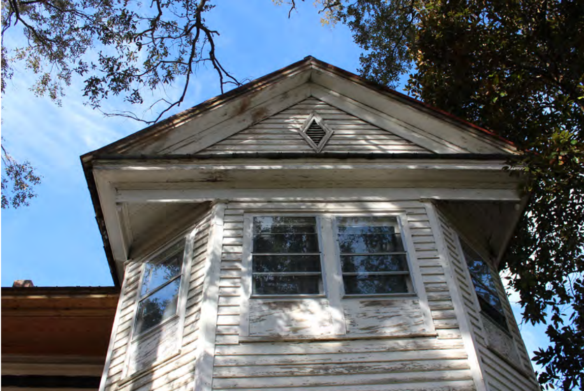
Figure 19: Epps-McGill Farmhouse - PHASE 01: Detail of cornice paint failure on the front facade (Kalen McNabb 2020).
