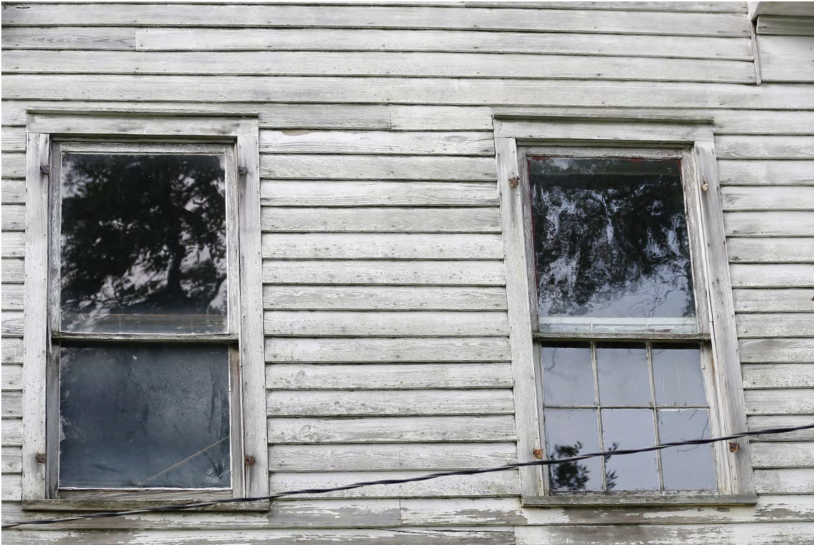
Figure 45: Epps-McGill Farmhouse - PHASE 02: View of window deterioration and haphazard replacement (Kalen McNabb 2020).
