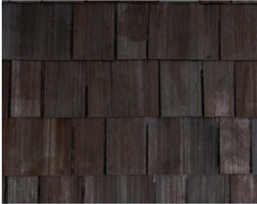
Figure 1: Epps-McGill Farmhouse - View of the Brava Cedar Shake in “Aged”.
