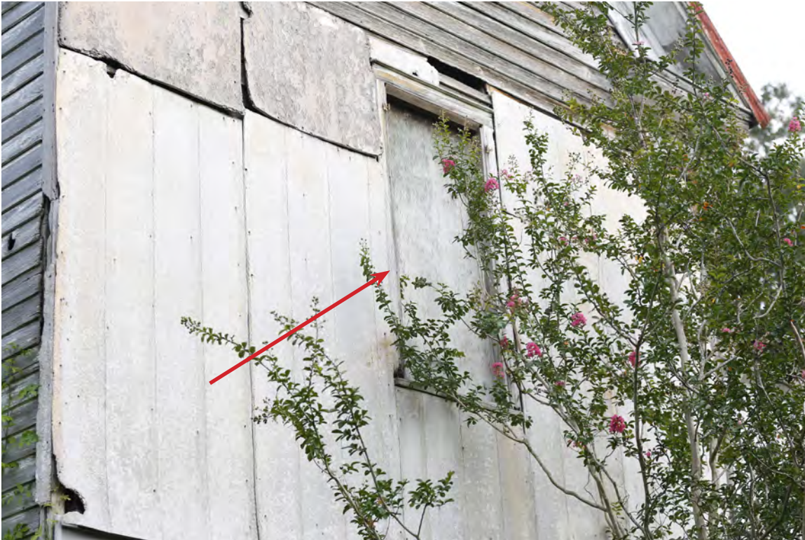
Figure 43: Epps-McGill Farmhouse - PHASE 02: Detail of missing sashes on the west elevation in a historic opening (Kalen McNabb 2020).
