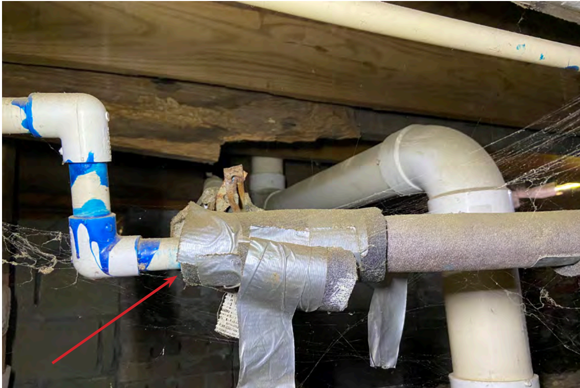
Figure 59: Epps-McGill Farmhouse - PHASE 02: Detail of leaking modern plumbing beneath the first-floor bathrooms (Kalen McNabb 2020).
