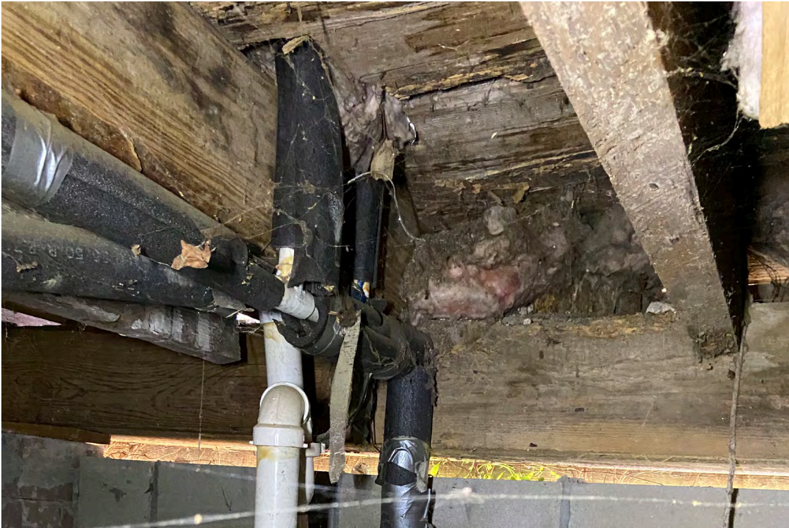
Figure 9: Epps-McGill Farmhouse - PHASE 01: Detail of framing deterioration beneath the first-floor bathrooms (Kalen McNabb 2020).
