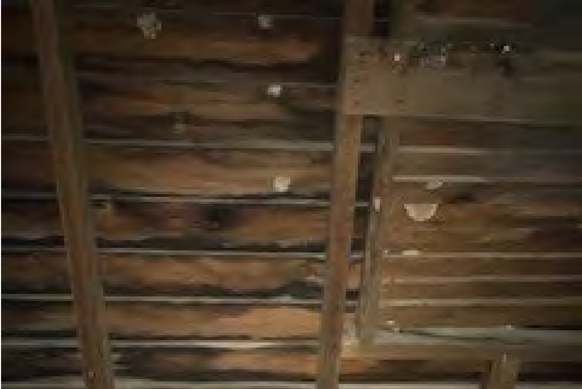
Figure 29: Epps-McGill Farmhouse - PHASE 01: Evidence of water intrusion is present on the historic sheathing (Kalen McNabb 2020).
