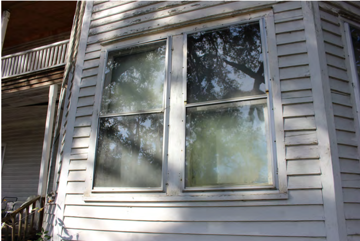
Figure 41: Epps-McGill Farmhouse - PHASE 02: Inappropriate storm windows have also been installed over many of the windows (Kalen McNabb 2020).
