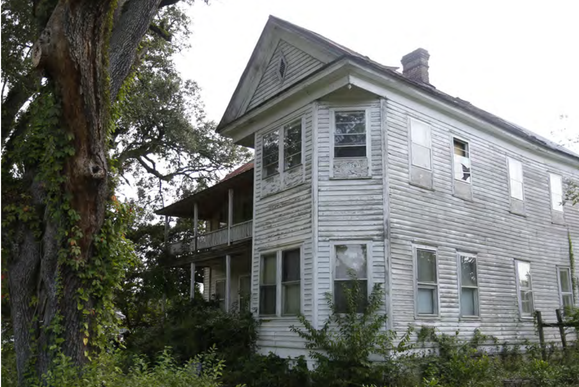
Figure 33: Epps-McGill Farmhouse - PHASE 02: The historic siding remains in place on 75% of the building and appears to be in fair condition (Kalen McNabb 2020).
