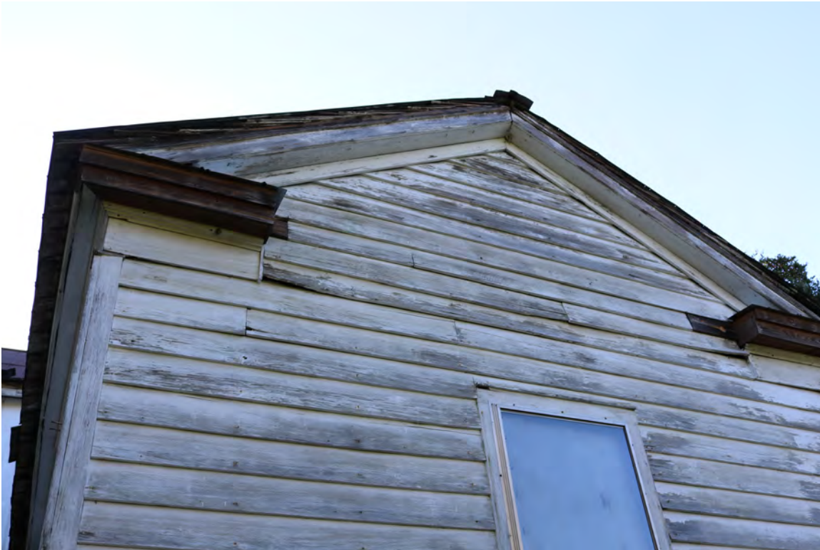
Figure 17: Epps-McGill Farmhouse - PHASE 01: The cornice has localized areas of wood deterioration and extensive paint loss on all cornice elements (Kalen McNabb 2020).
