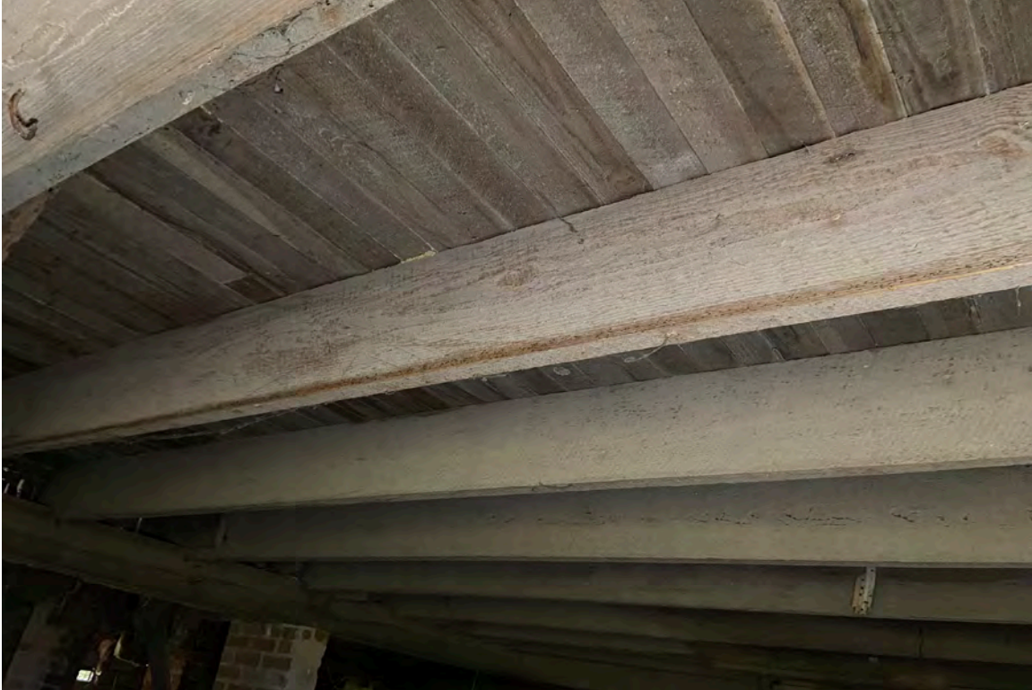
Figure 7: Epps-McGill Farmhouse - PHASE 01: The historic joists are in good condition with isolated areas of failure requiring intervention (Kalen McNabb 2020).
