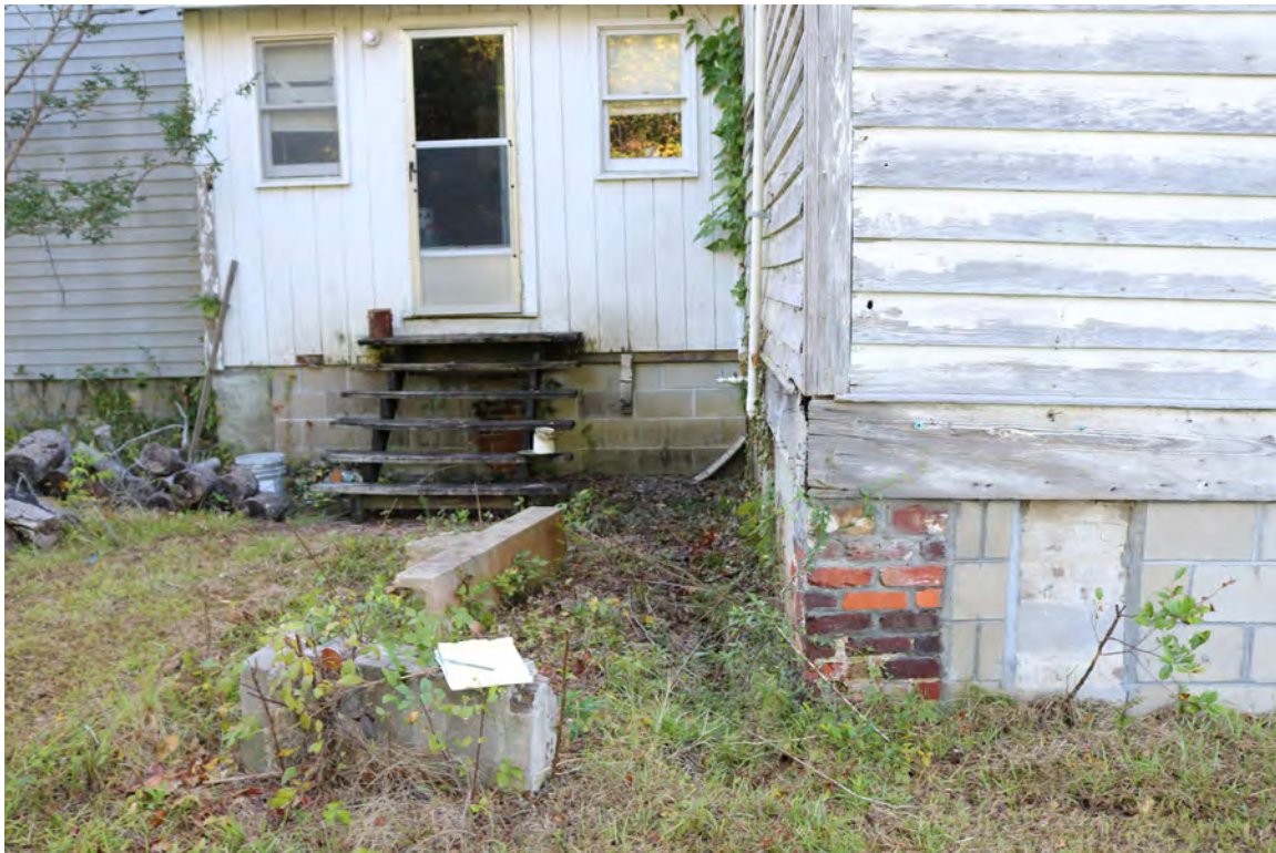
Figure 54: Epps-McGill Farmhouse - PHASE 02: View of location of deck and ramp. The existing modern wood stair is deteriorated and lacks a railing (Kalen McNabb 2020).
