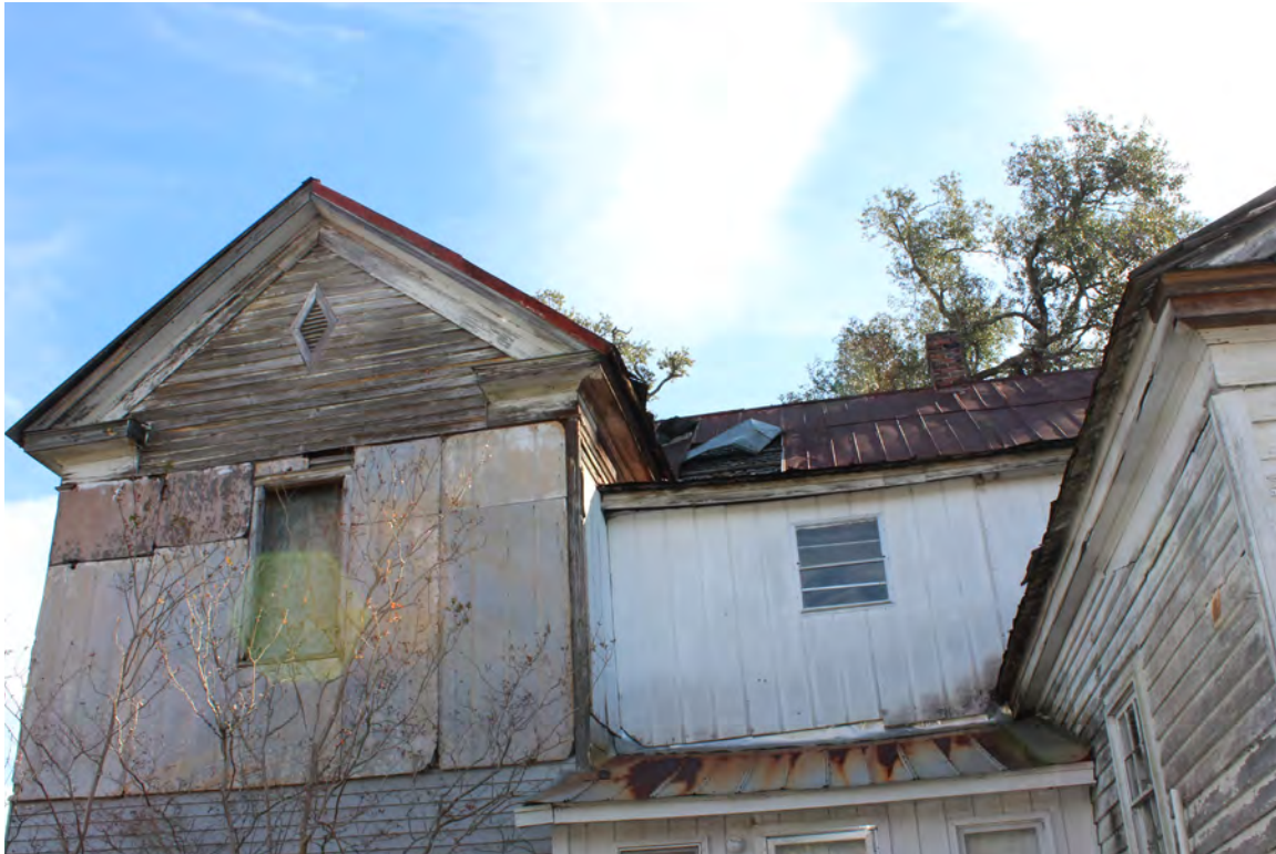
Figure 37: Epps-McGill Farmhouse - PHASE 02: Overview of the mixture of siding materials on the west elevation (Kalen McNabb 2020).
