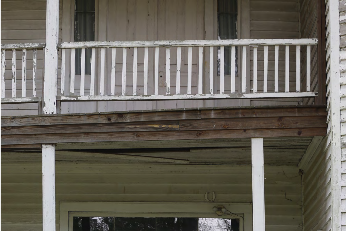
Figure 15: Epps-McGill Farmhouse - PHASE 01: Detail of Porch Railing Failure (Kalen McNabb 2020).
