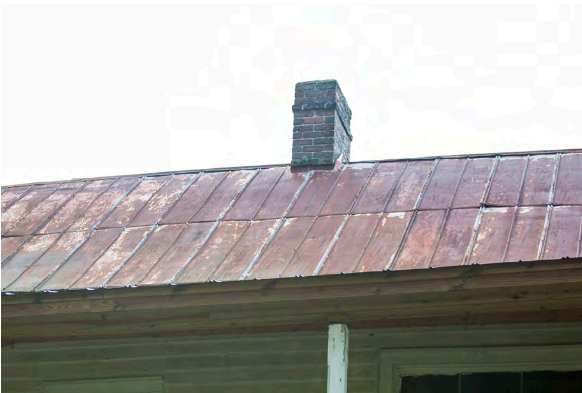
Figure 25: Epps-McGill Farmhouse - PHASE 01: The chimneys are in fair condition but likely require repointing (Kalen McNabb 2020).
