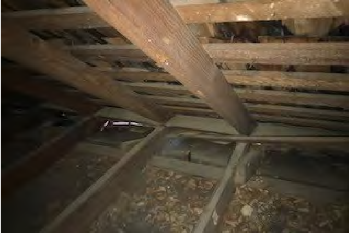
Figure 27: Epps-McGill Farmhouse - PHASE 01: The attic framing is in fair condition but the wooden framing members are undersized and over-spanned (Kalen McNabb 2020).
