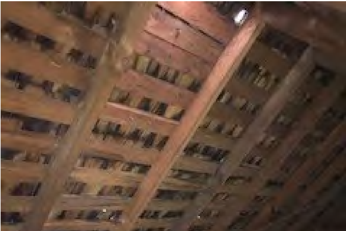
Figure 28: Epps-McGill Farmhouse - PHASE 01: The rafters are deflecting and require additional support (Kalen McNabb 2020).
