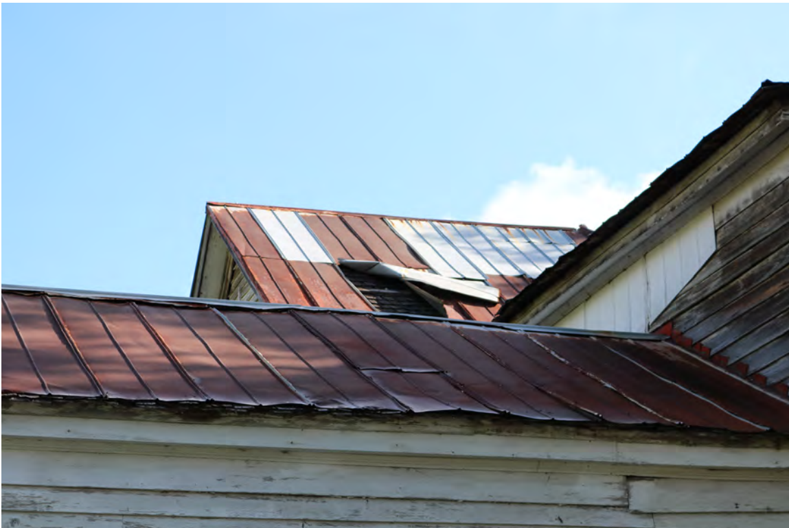
Figure 22: Epps-McGill Farmhouse - PHASE 01: Many of the metal roofing panels are detaching (Kalen McNabb 2020).
