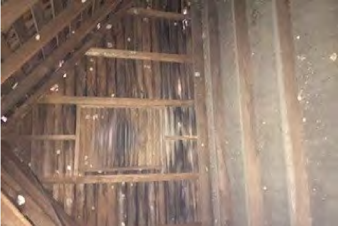
Figure 31: Epps-McGill Farmhouse - PHASE 01: The ceiling joists are also over-spanned and undersized (Kalen McNabb 2020).
