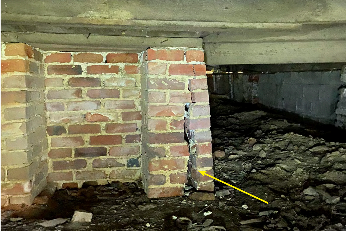
Figure 3: Epps-McGill Farmhouse - PHASE 01: The north foundation chimney is cracked (Kalen McNabb 2020).
