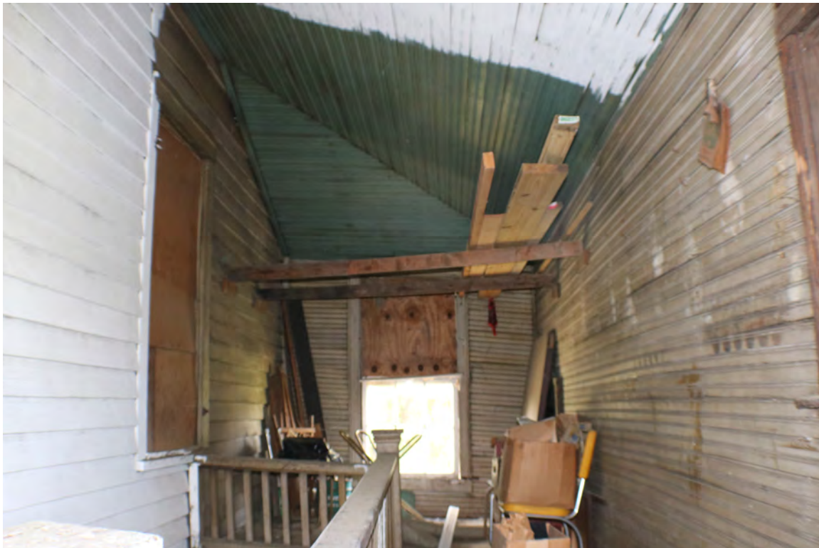
Figure 70: Epps-McGill Farmhouse - PHASE 02: View of extant beadboard. All historic woodwork will be preserved (Kalen McNabb 2020).
