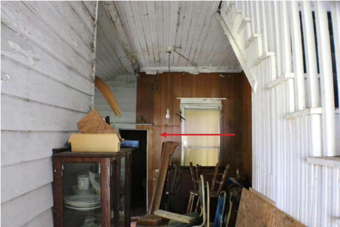
Figure 61: Epps-McGill Farmhouse - PHASE 02: View of existing opening to be reused for the half bathroom Room 109. The window infill to remain (Kalen McNabb 2020).
