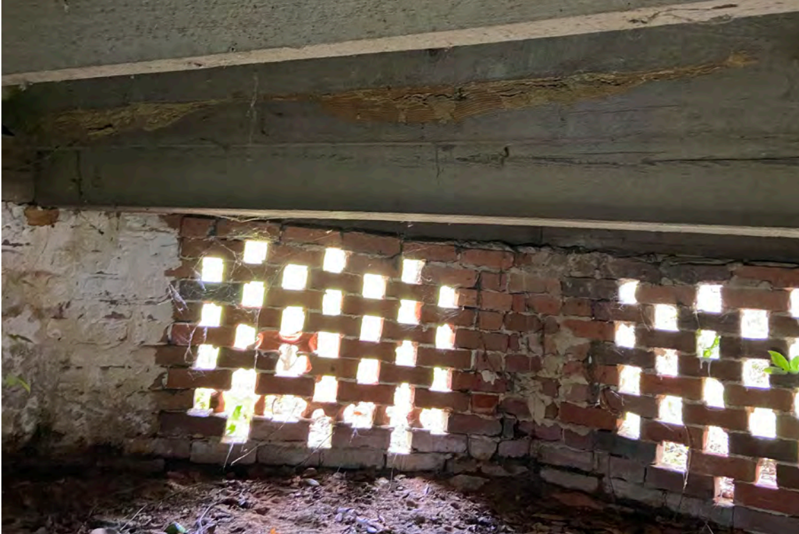
Figure 5: Epps-McGill Farmhouse - PHASE 01: Select areas of the foundation require repointing (Kalen McNabb 2020).
