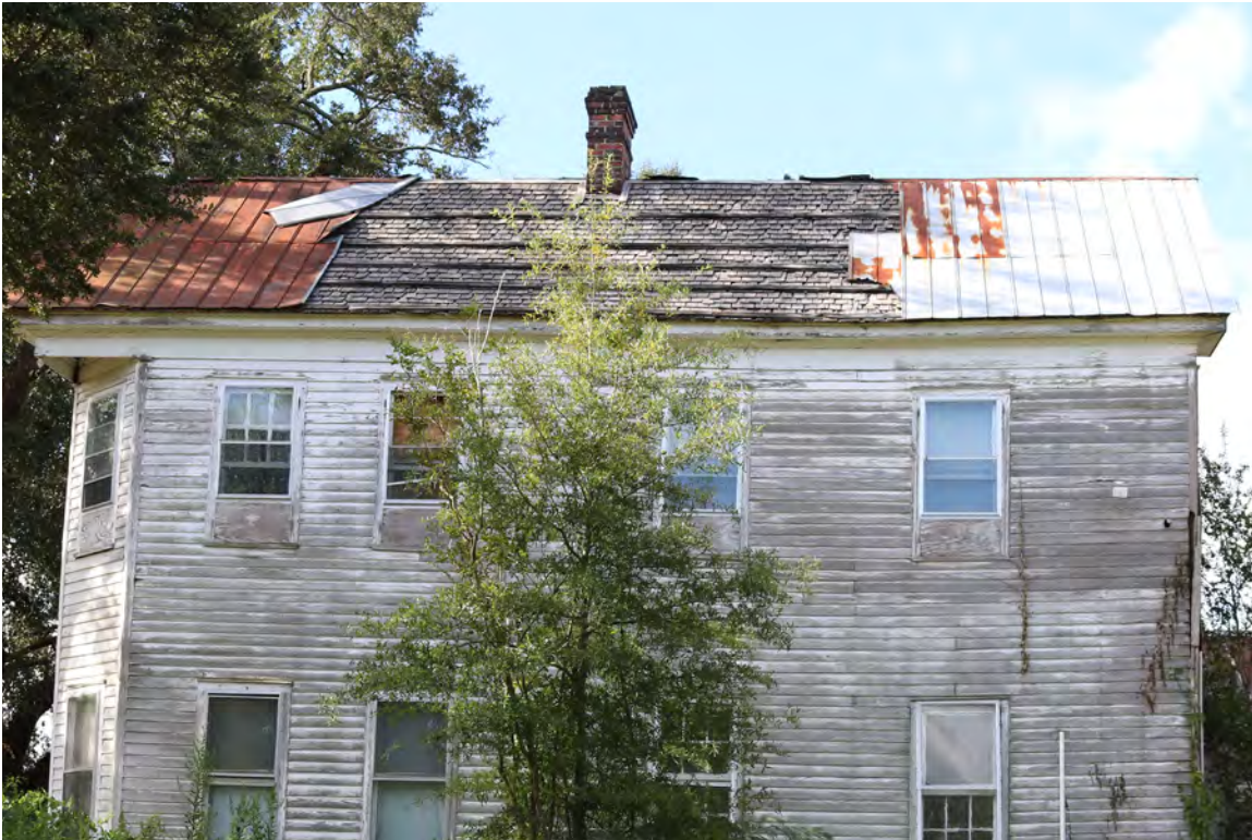
Figure 21: Epps-McGill Farmhouse - PHASE 01: The existing 5V metal roof is heavily corroded and missing on 30-40% of the roof. (Kalen McNabb 2020).
