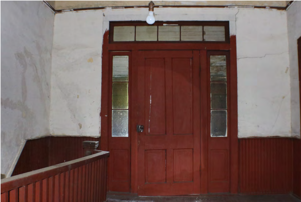
Figure 47: Epps-McGill Farmhouse - PHASE 02: View of original second-floor porch door (Kalen McNabb 2020).
