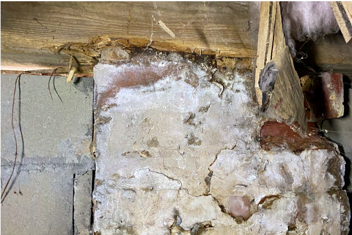
Figure 2: Epps-McGill Farmhouse - PHASE 01: Detail of masonry deterioration and efflorescence (Kalen McNabb 2020).
