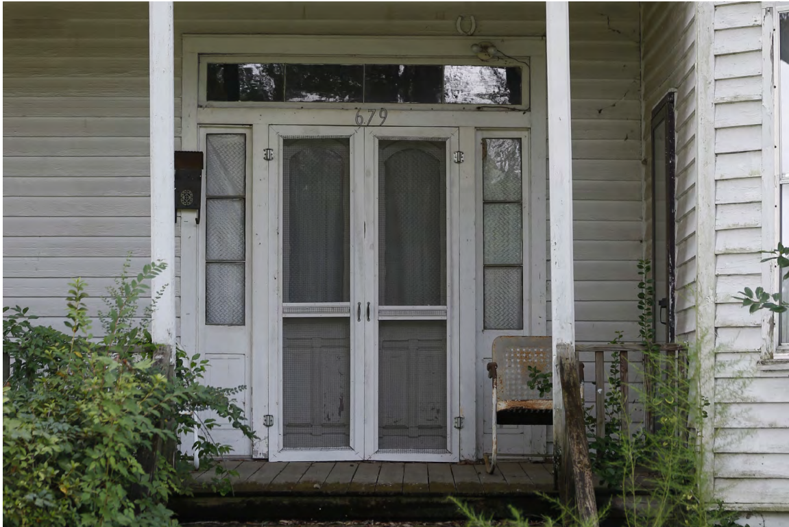
Figure 39: Epps-McGill Farmhouse - PHASE 02: The front doors are in good condition but require restoration (Kalen McNabb 2020).
